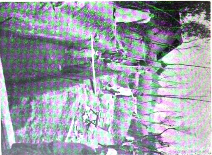
The first trench when nearly completed. The water from the big irrigation ditch was later turned into this trench and the ditch pumped dry.
